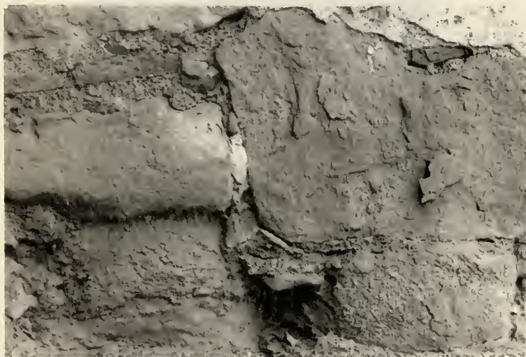
Fig. 22. Flaking of green sandstones above base of wall at north wall of east transept.
